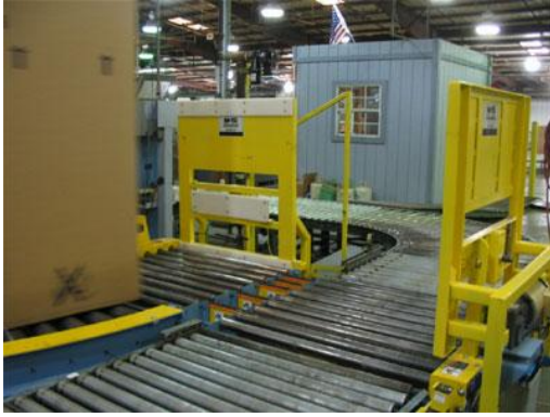
Crossover roller conveyor system
